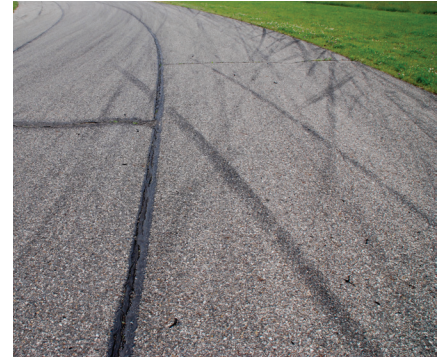
The 20-year-old track pavement was intact, but there were 1 ½-inch cracks that had been filled with rubber crack seal.
